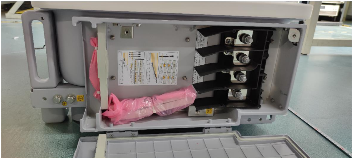
Photo-20: AC connection compartment
